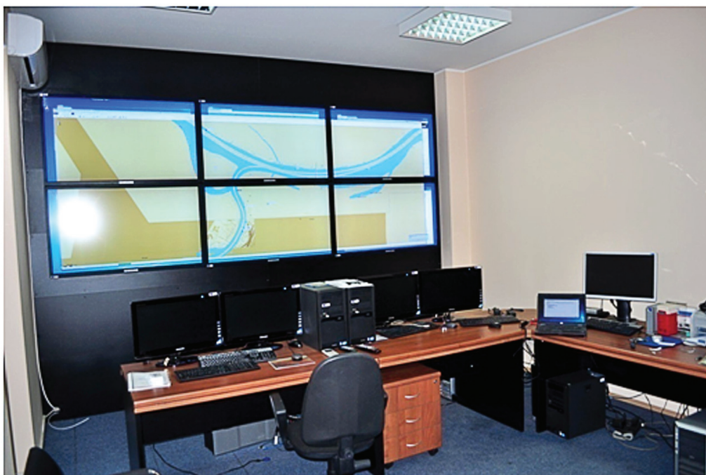
Figure 90. The national RIS centre – control room
